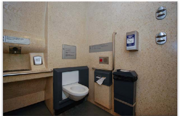
Wall mounted contaminated sharps container
